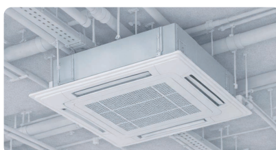
Refrigerant gas detection for air conditioning equipment
